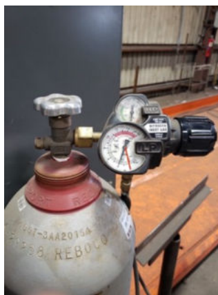
Figure 16 – RTW 3.0 Pressure Regulators Leaks
