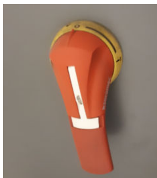
Figure 57 – RTW 3.0 Main Power Switch
