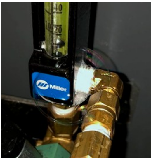
Figure 15 – RTW 3.0 Gas Flow Meter Leaks
